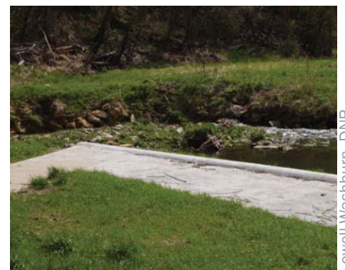
Below: A section of the sidewalk that provides fishing access to Grannis Creek for people with disabilities.
