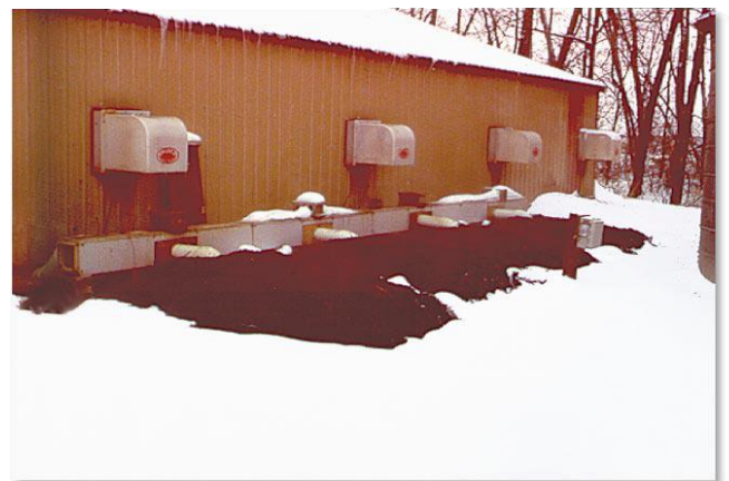
Installed biofilter at a swine facility.
