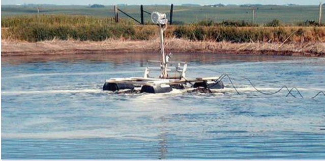
Aerator on second-stage lagoon at swine facility will reduce hydrogen sulfide emissions, but may also increase ammonia emissions.
