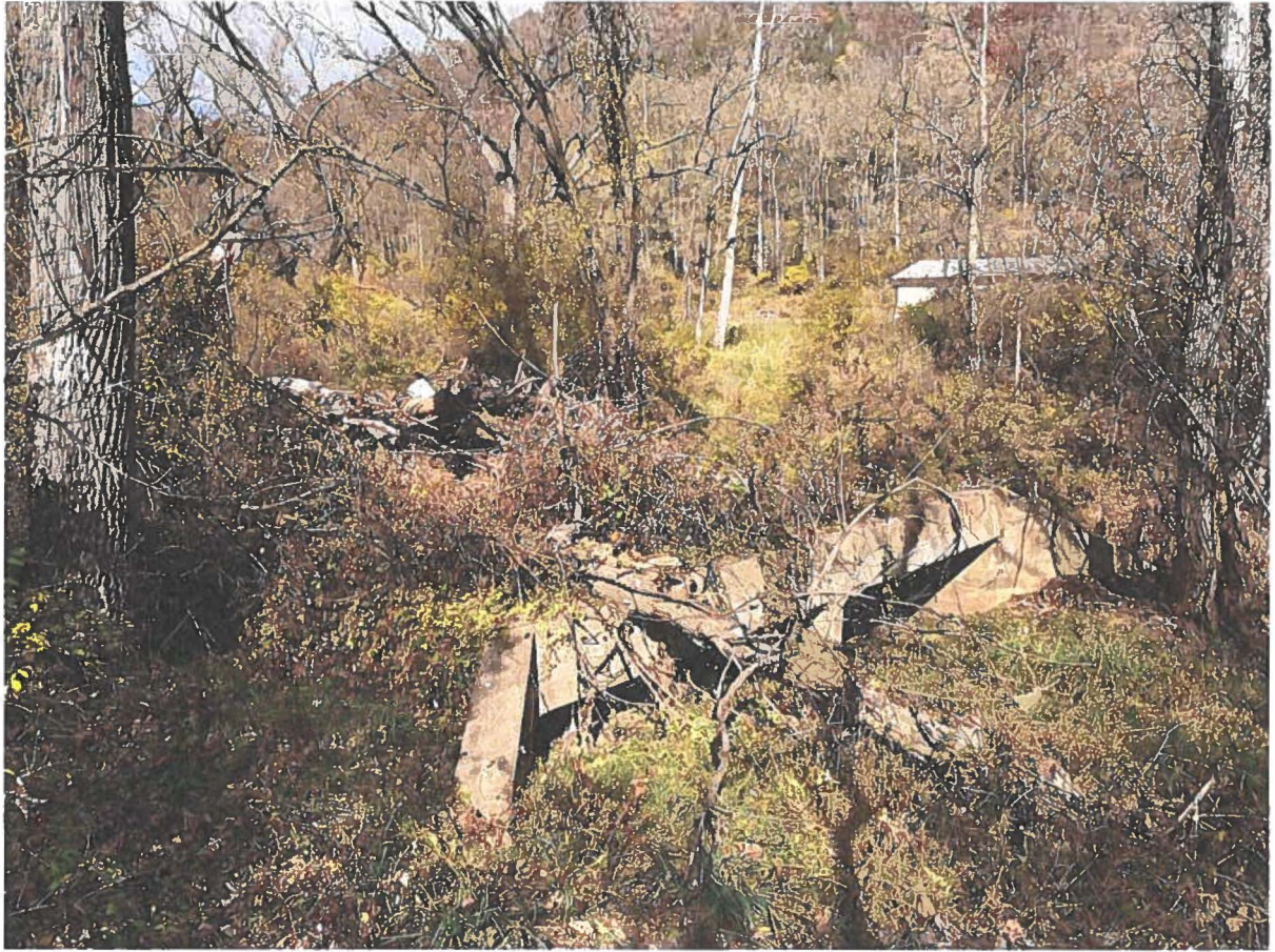
Overhead photo of concrete culvert – downstream side with log jam at the top left of photo
