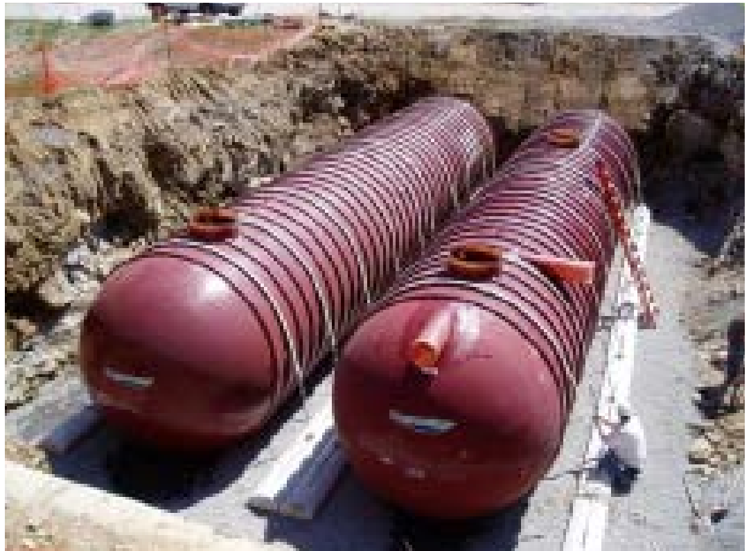
FRP below ground storage tanks with anchoring. Image courtesy of Watertronics.
