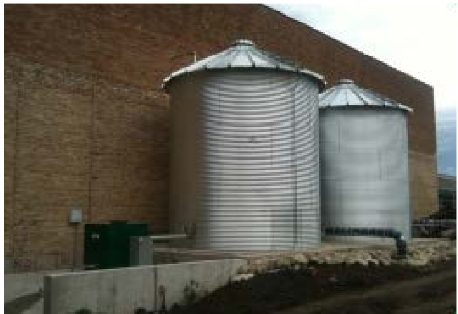
Corrugated metal tanks. Image courtesy of Watertronics.
