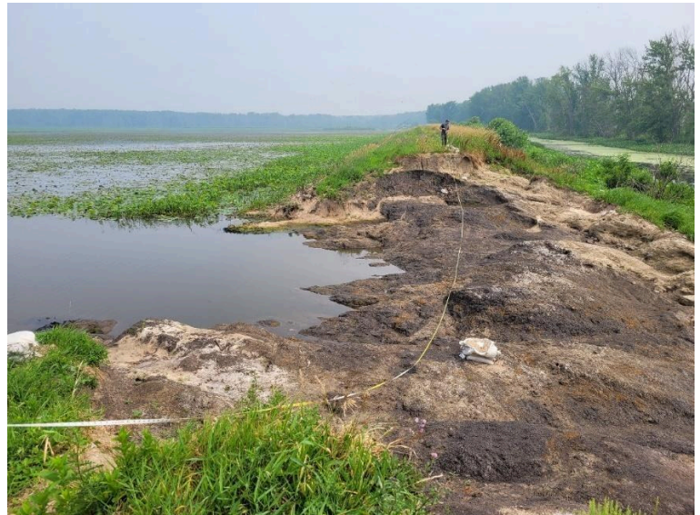
Damage at Main Levee in Green Island Wildlife Management Area
