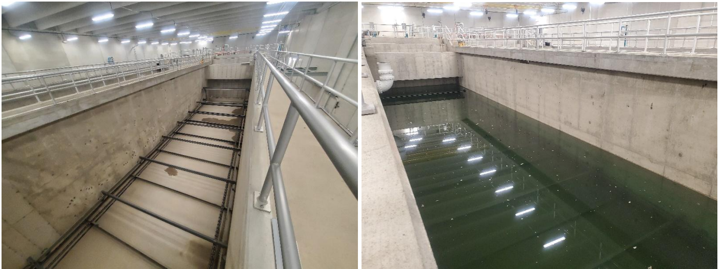
Sedimentation basins of a new surface water treatment plant, constructed primarily in 2025 using DWSRF funds. The empty sedimentation basin on the left displays the sludge collection system on the bottom.
