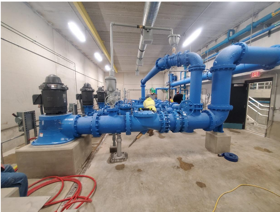
High service pumps moving water from clearwells to the distribution of a surface water treatment plant.
