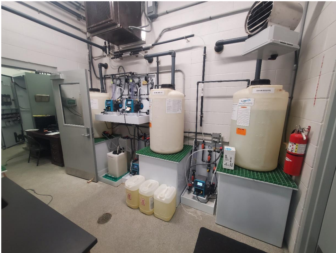
Chemical storage room of a surface water treatment plant.
