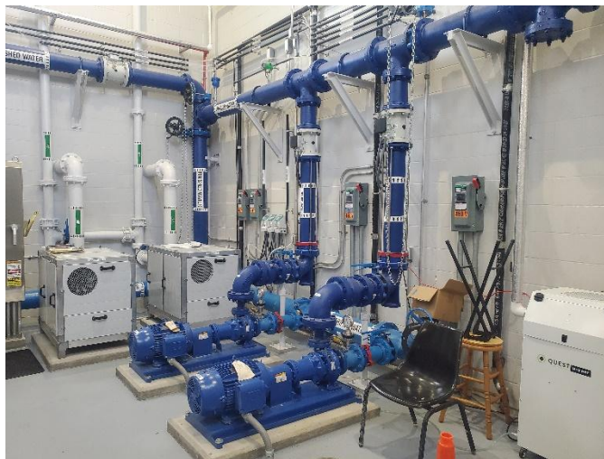
Blue high service pumps and blowers in a groundwater treatment plant.
