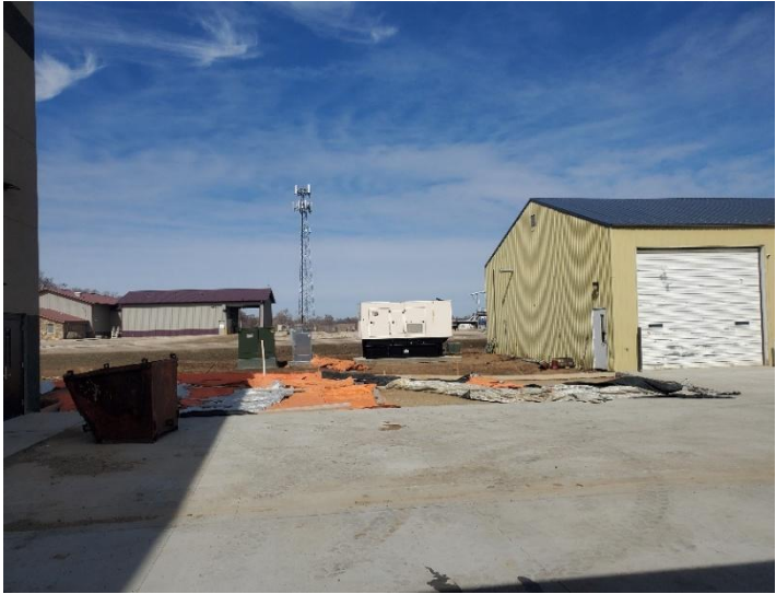
New generator installed outside a treatment plant, providing backup power in the event of an outage.
