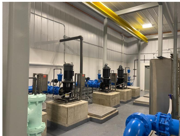
High service pumps to distribution system
