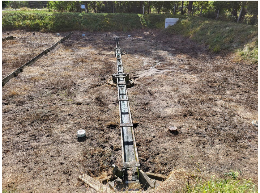
Existing Sand Filter
