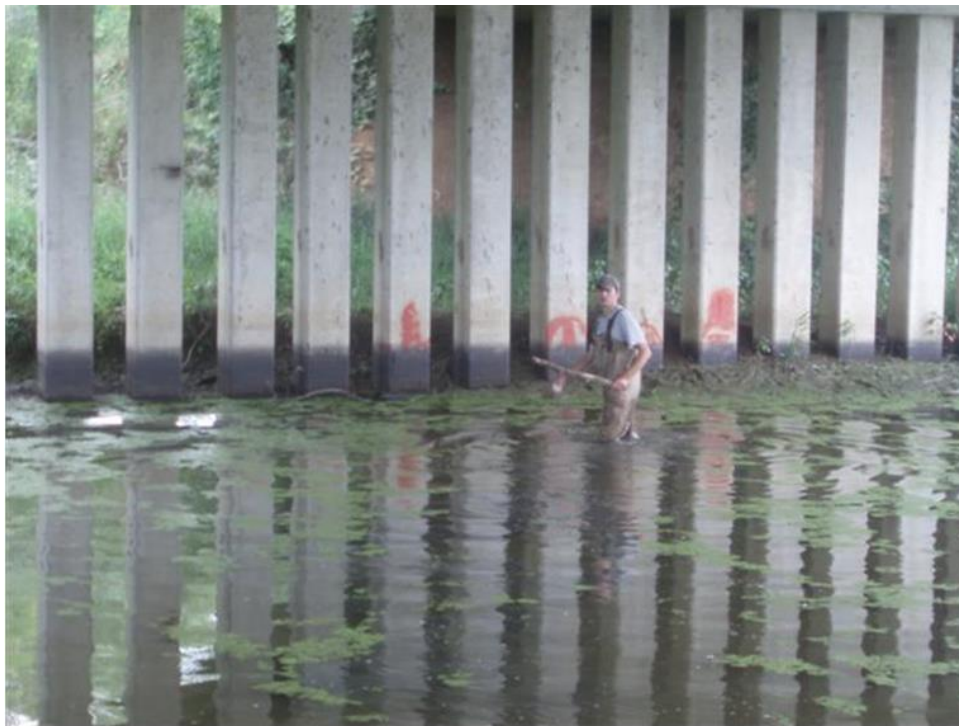
Figure 34. 614-2 Graffiti present under the bridge.
