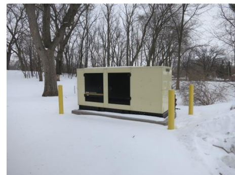
Major Monitoring & Reporting Violations
