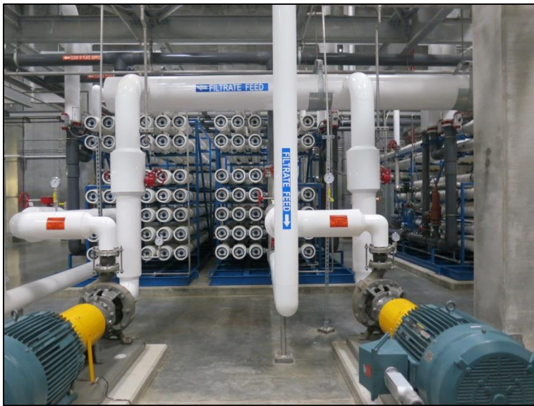
Reverse osmosis skids with pumps.
