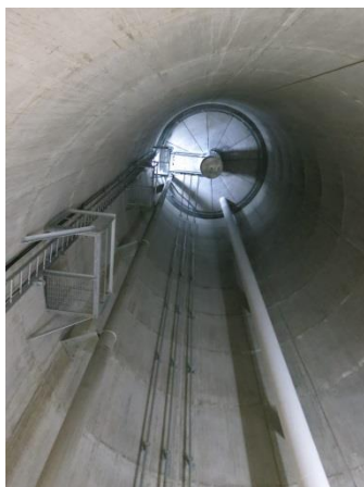
View of the underside of the elevated storage tank within the pedestal
