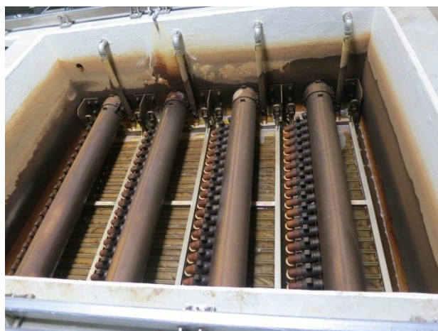
An ultrafiltration treatment unit
