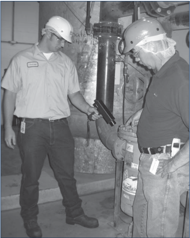
Andrew Engle and Jim Wernet use an ultrasonic detector to measure an air leak at the Kraft plant.
