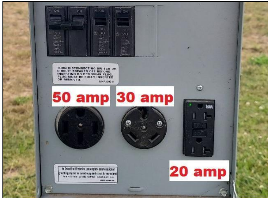
Photo of the electricity box
