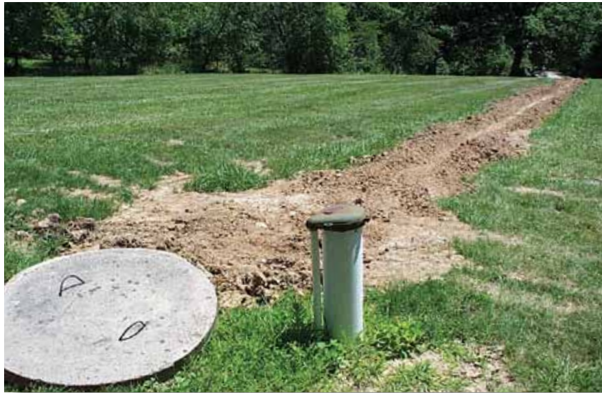
New construction of a wellhead with grass and trees planted in the capture zone.
