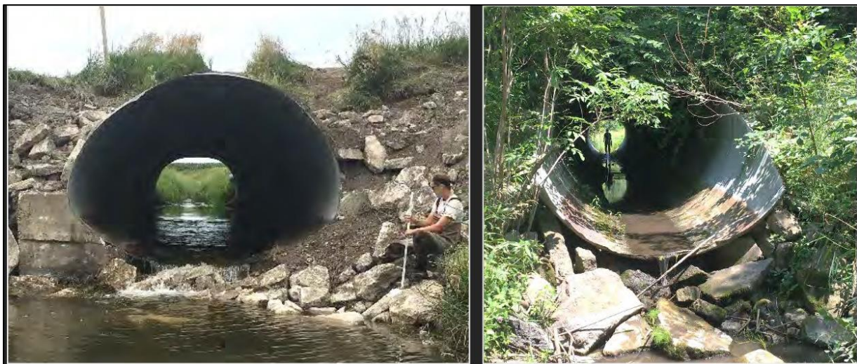
Figure 32: Example of Perched Culverts within the Boone River Watershed (Jarvey, 2021)
