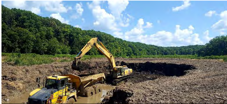
Mechanical dredging of excess soft sediments at Lake Geode help improve overall water quality and recreational opportunities in the lake.
