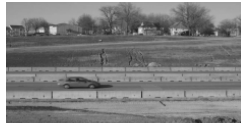
Example of rills caused by exposed subsoil not treated with compost along I-235.
