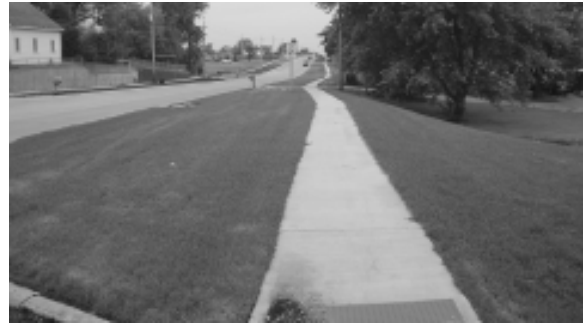
View of extensive work along Locust Street; note the second application of compost on the left side of the street.
