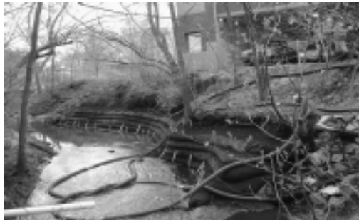
Application of compost at ISU to stabilize stream near a parking structure in April 2004.
