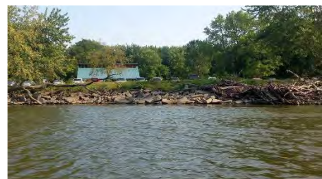
Broken concrete and fallen branches define the shoreline near the boat ramp
