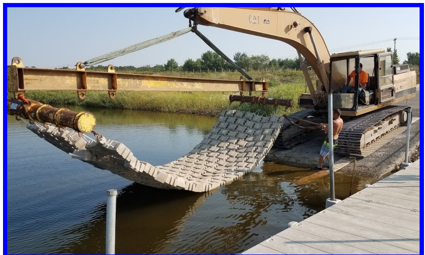
The west boat ramp lane at West Lake Osceola was extended this summer through the addition of sections of ArmorFlex concrete pads. Photo by: Jason Kruse (DNR Engineering)
