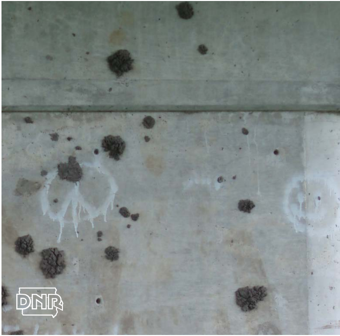
Evidence of Human Use – Evidence of Kids Play Drawings & mud balls under bridge
