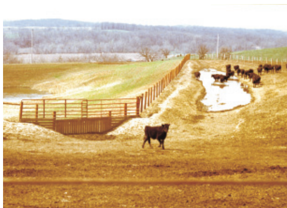
Solids settling structure with slotted gate.
